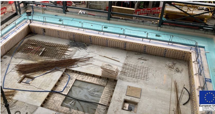
Steel frame ready for cladding, while insulation is added to the chamber pits © Richard Fitton
